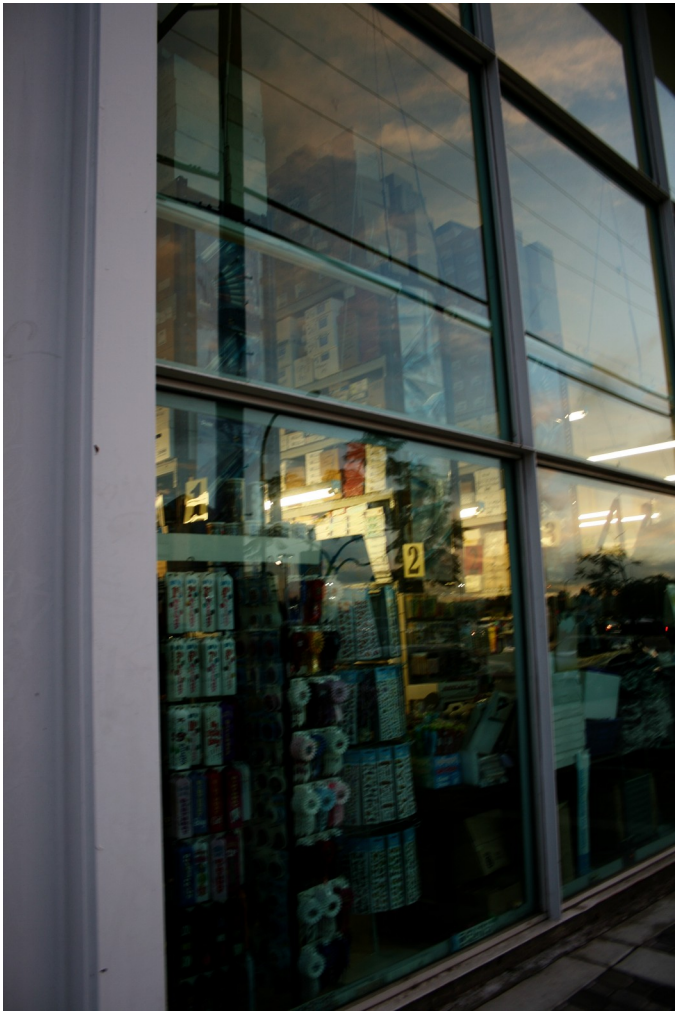
Suspected hazardous fire conditions
